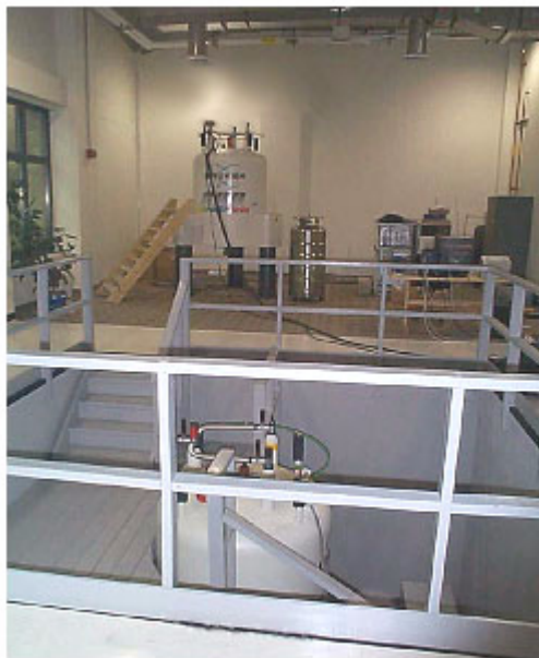
Figure 5.4. Example of a Magnet Pit
