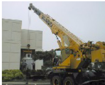
Lifting the magnet and positioning it on air-skates in front of the access doors to the building.
