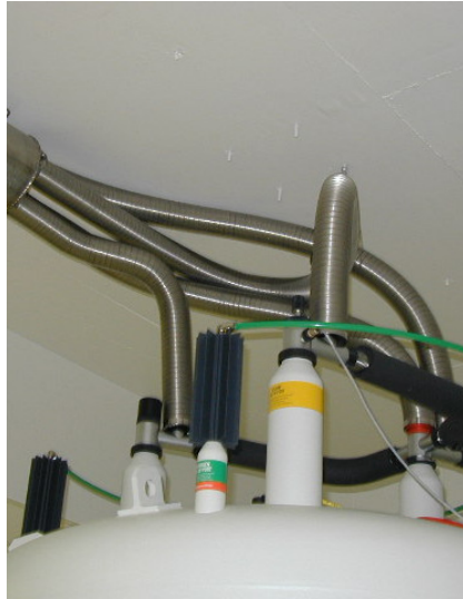
Figure 8.2. Emergency Quench Pipes
